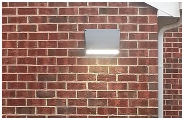
Exterior-Installed LED Lights
